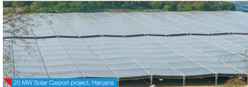
20 MW Solar Carport project, Haryana
