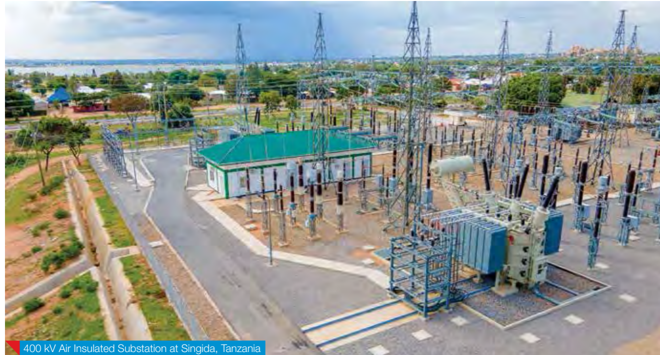
400 kV Air Insulated Substation at Singida, Tanzania
