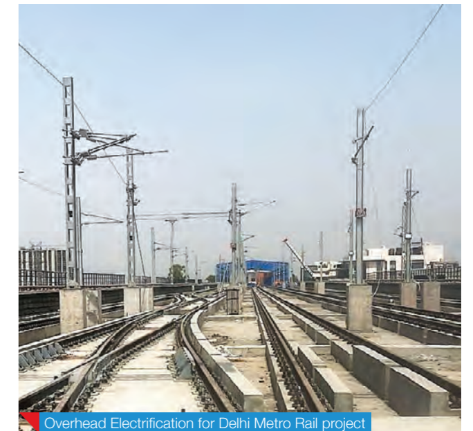
Overhead Electrification for Delhi Metro Rail project
