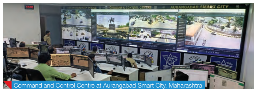
Command and Control Centre at Aurangabad Smart City, Maharashtra
