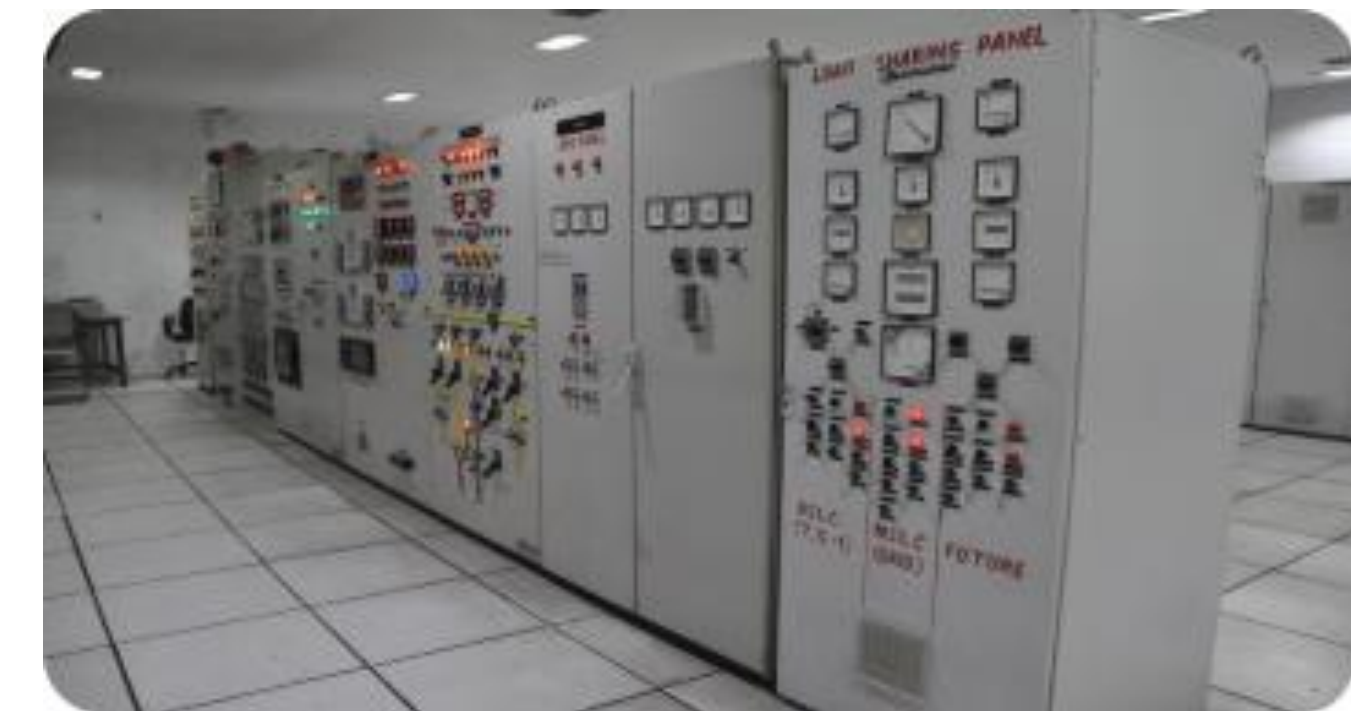
Cogeneration Control Panel
