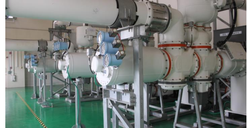
Commissioned 132/11KV GIS Sub-Station for auto major in Rhotak, Haryana
