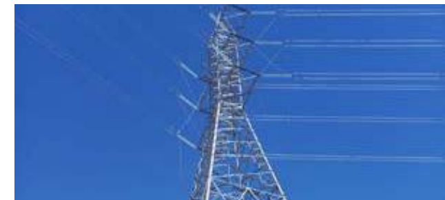
220 kV - D/C Tower
