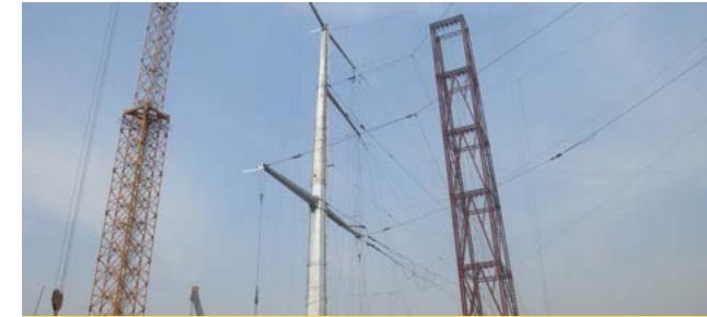
765 kV S/C - Monopole
