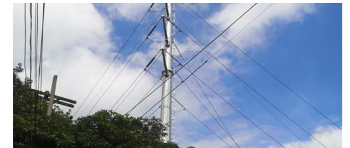
500 kV D/C - Tower
