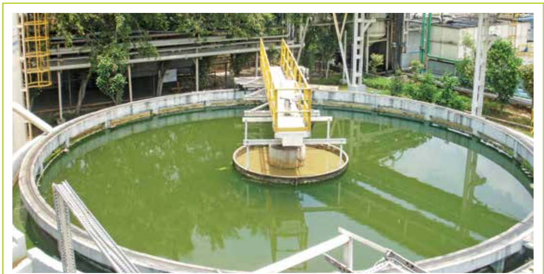
Effluent treatment plant at Gurugram facility
