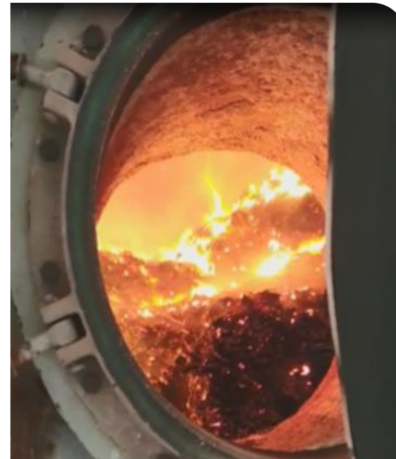
Efficient combustion (without support fuel)
