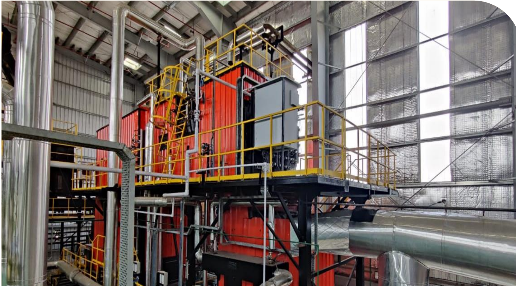
16TPH Steam boiler for curing of rubber
