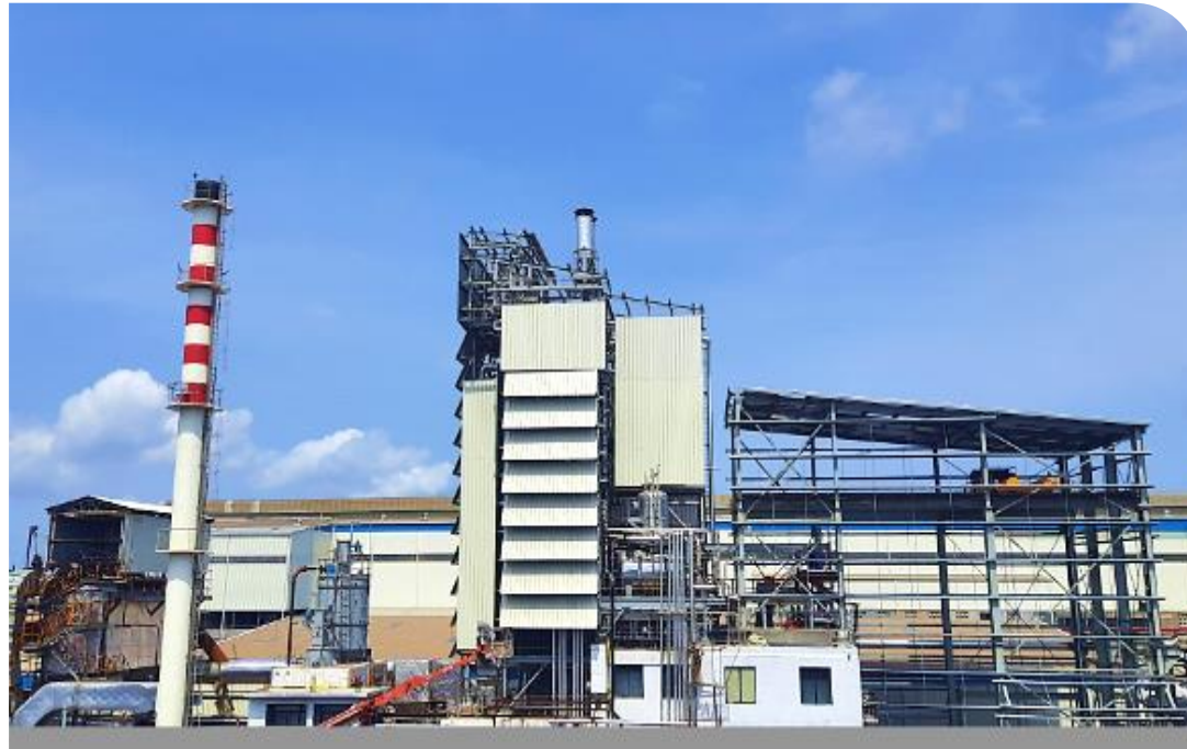
14TPH Non-Recyclable Solid Waste (NRSW) fired boiler
