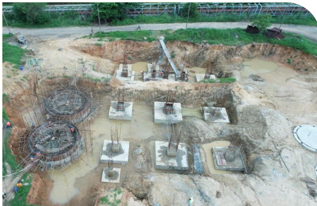
FGD- Flue gas desulfurization
