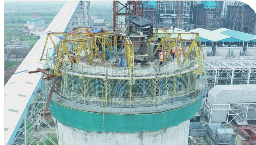
Wet Stack at 60 mt
