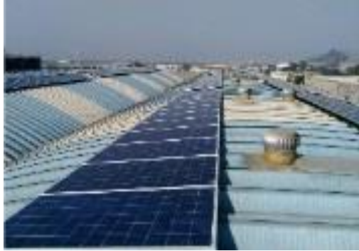
Rooftop mounted solar system
