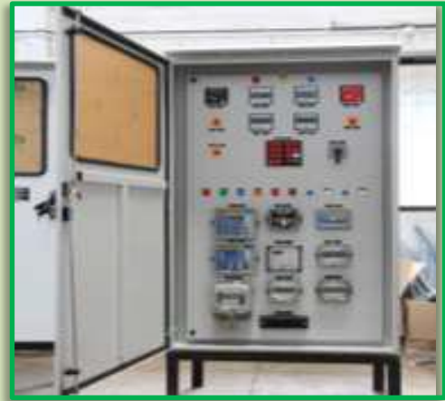
Control and Relay Panels
