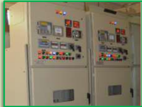
Indoor MV Switchgears upto 33 kV
