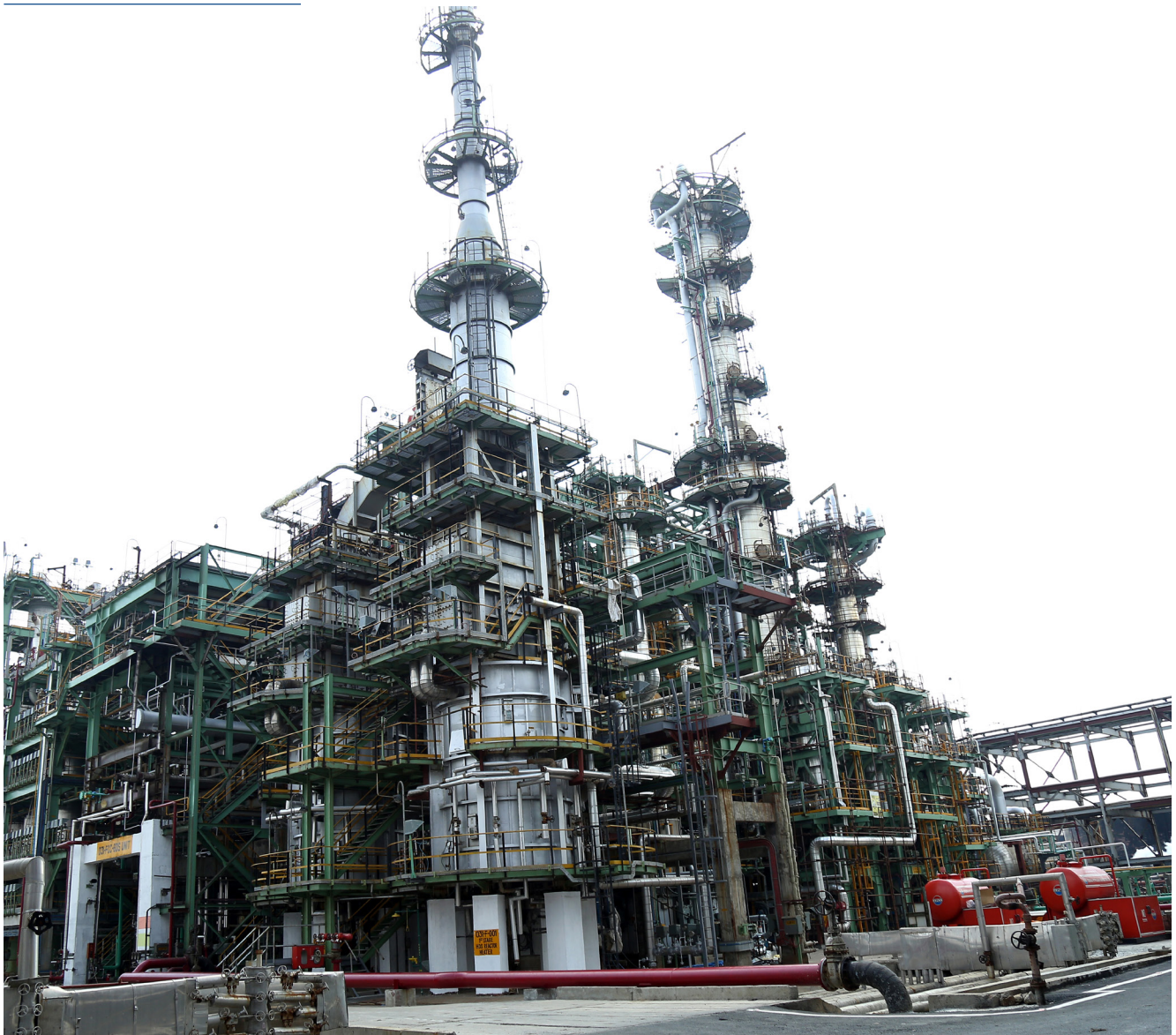
FCC-GDS, FCCU Flare system switched over to Demountable Flare and commissioned on 12.08.21 and 20.08.21, respectively
