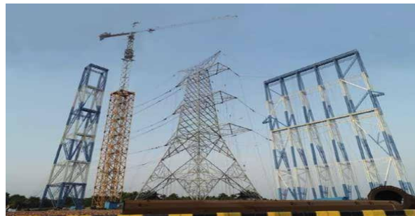
765kV Transmission Tower
