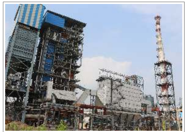
Thermal Power Plant - Durg
