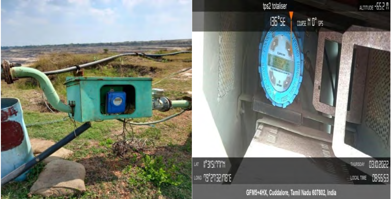
Flow Meters Installed
