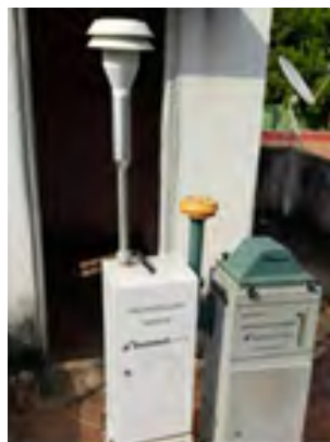
AAQ Station installed in Mudhanai, Neyveli
