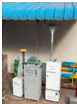
AAQ Station installed in Vadakuvellore, Neyveli
