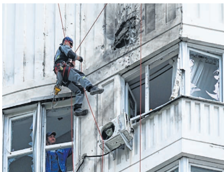
A specialist inspects the damaged facade of a multi-storey apartment after reported drone attack in Moscow on Tuesday
