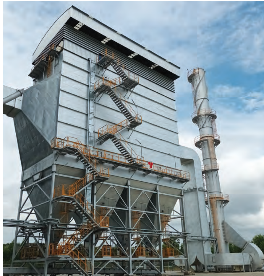
Thermax has installed an electrostatic precipitator (ESP) for a power company in Thailand to control emissions from their 26 MW biomass power plant
