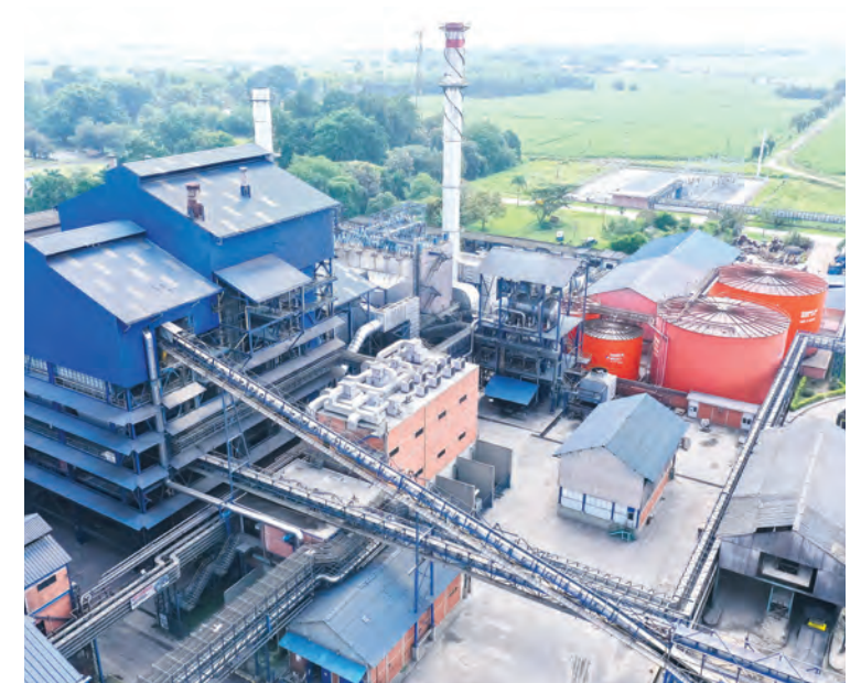
250 TPH boiler installed for a customer in Columbia
