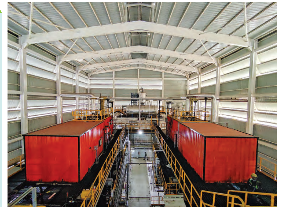
State-of-the-art biomass based boiler plant set up for a leading food major
