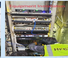
Fiber Optic Transmission System - FOTS
