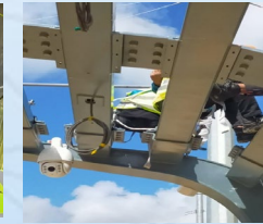
CCTV Video Surveillance System
