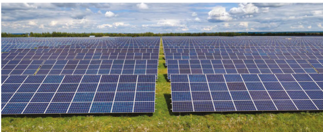
Group Captive Solar Power projects for Ennore and Mangalore have been commissioned in March 2024
