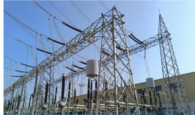
Jauljibi Substation, Uttarakhand
