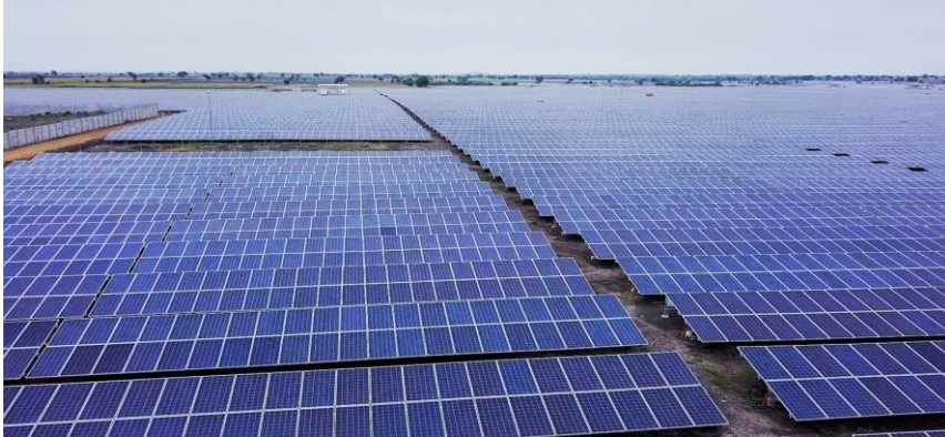
100 MW (AC) Solar Plant (Reduces 200mn kg CO 2 emissions annually)
