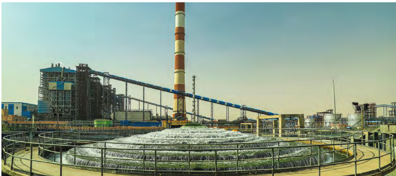
2x660 MW super critical power plant under commissioning by BHEL at Suratgarh, Rajasthan
