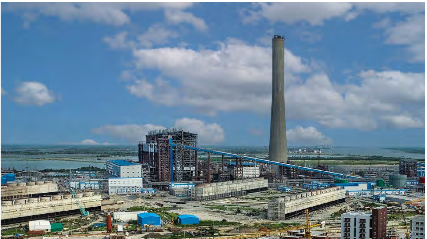
2x 660 MW Maitree Supercritical Power Project being executed by BHEL in Bangladesh
