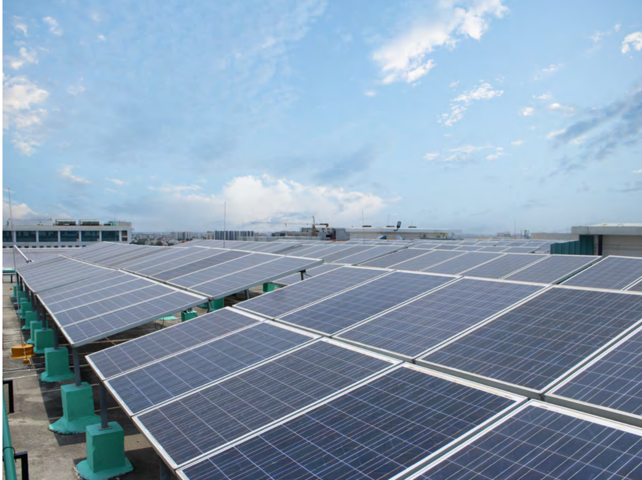
▲ Solar Panels installed at DLF Cybercity, Chennai
