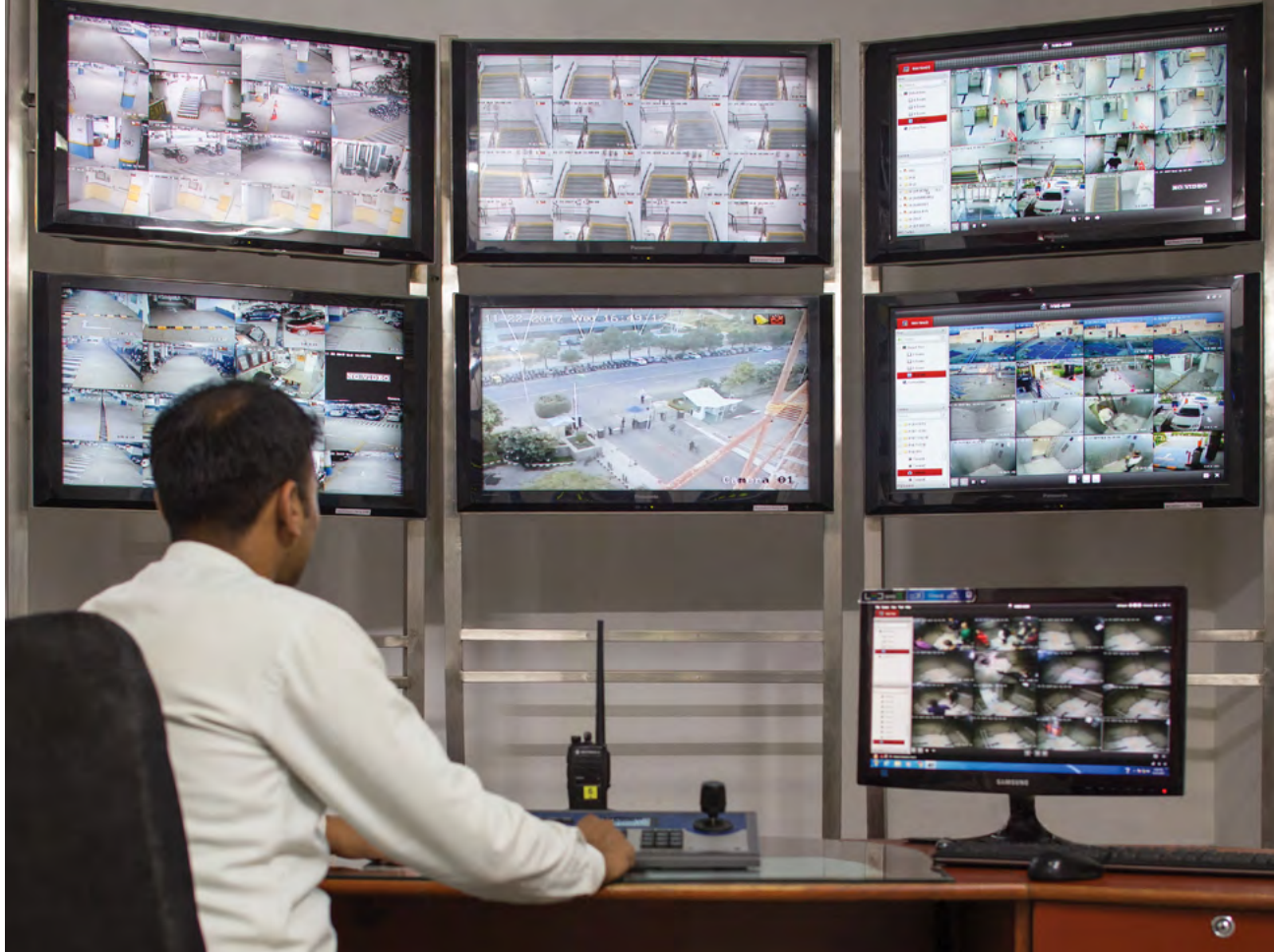
▲ CCTV Monitoring at our facility
