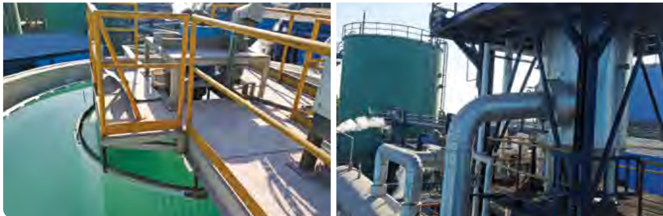
Effluent Treatment Plant (ETP) at Mundra, Gujarat
