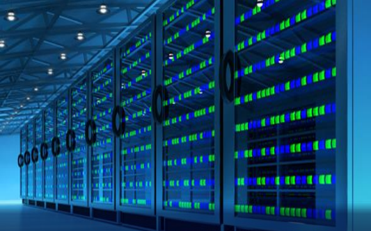
Data Center electrification with high efficiency, reliability and safety
