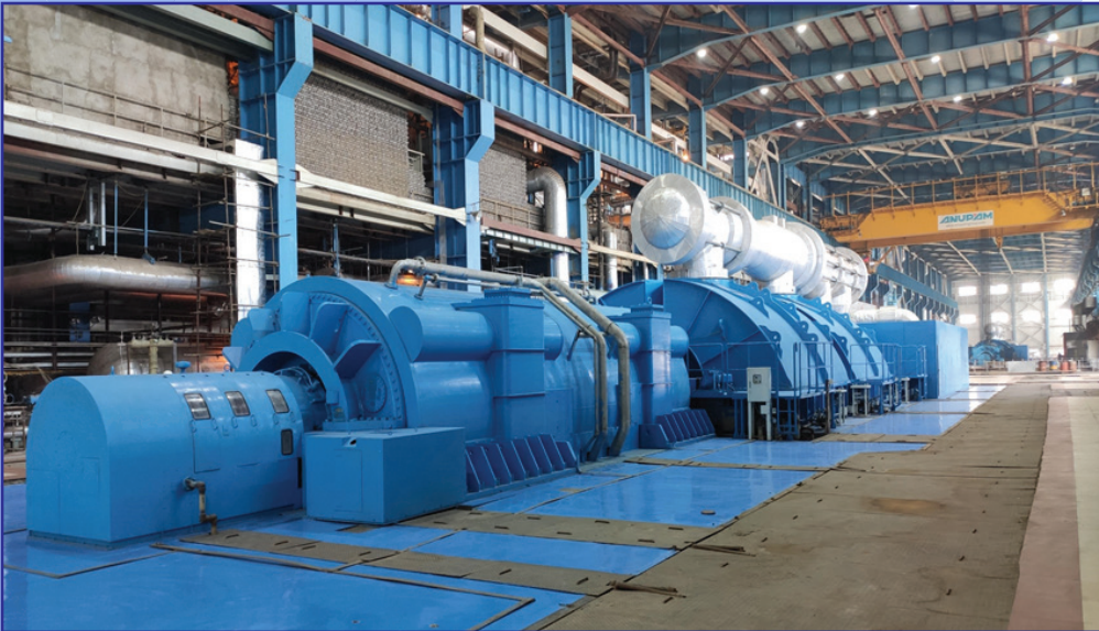
UNIT #2 NTPC 2x800 MW LARA STPP
