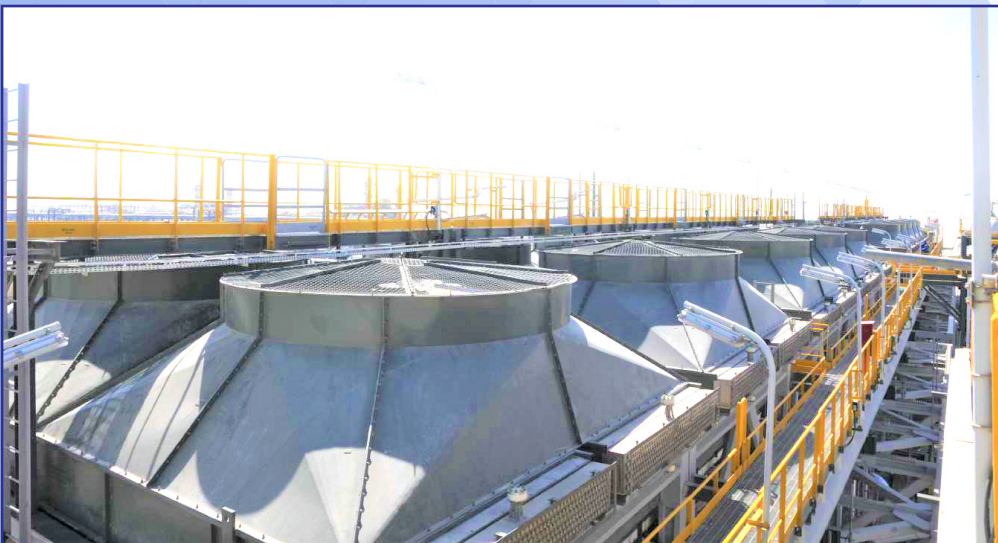
AIR COOLED HEAT EXCHANGERS INSTALLED AT HABSHAN-5 GAS FIELD OF ADNOC, ABU DHABI
