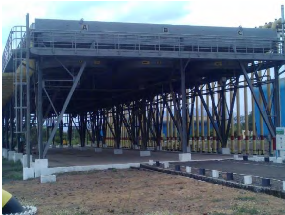
CS - 8 Gas After Cooler
