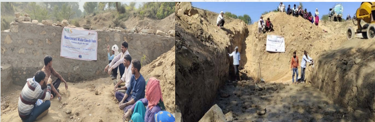
Check dams being constructed in Alwar district to catch and channelize rain water. Another sustainable initiative is to channelize and save water through a project of "Water conservation through installation of rainwater harvesting structures in the form of check dams and gabion structures" in Alwar, Rajasthan. PFS has funded four check dams and two gabion structures to improve ground water situation in the area.
