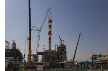
1519 MW FADHILI COMBINED HEAT AND POWER (CHP) PLANT KSA
