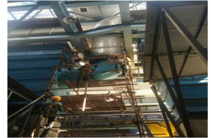
MSH LINE MODIFICATION, 600 MW SINGARENI
