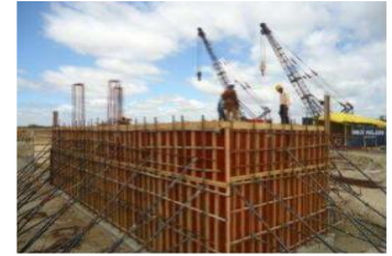
1X110 MW, CIVIL AND STRUCTURAL WORKS ,R&M OF MAIN PLANT, BATHINDA, BHEL
