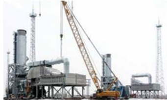
35 MW GT POWER PLANT, KAZAKSTHAN
