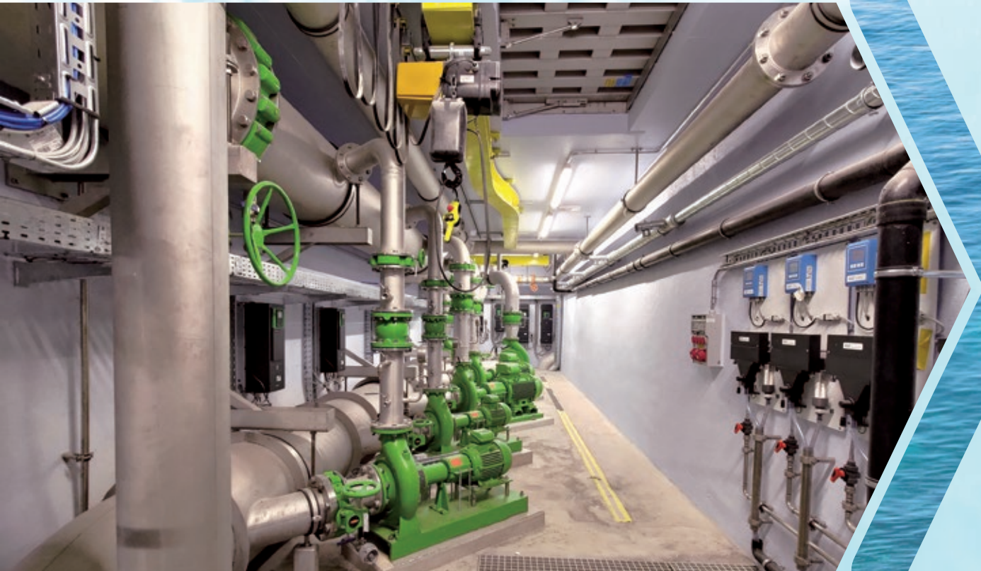
Lake water works Champ Bougin, Neuchatel, Switzerland
