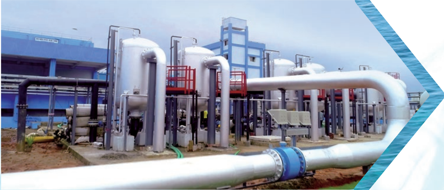
Koyambedu TTRO Plant, India
