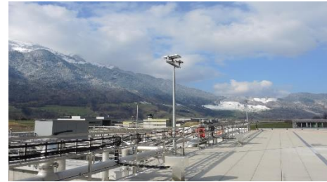
14 Sarneraatal WWTP, Alpnach, Switzerland First plant in Switzerland to be commissioned with NEREDA® technology
