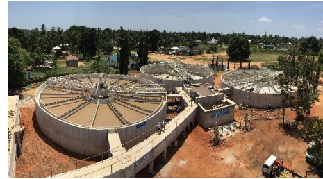
130 MLD Drinking Water Treatment Plant, Tanzania First water project in Africa to be commissioned under EXIM India funding
