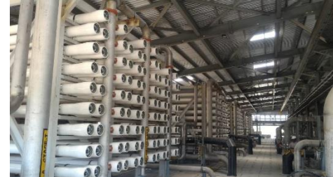
50 MLD BWRO (Desalination), for Reliance Industries, Dahej, India Turnkey project executed in record 8 months 24 days
