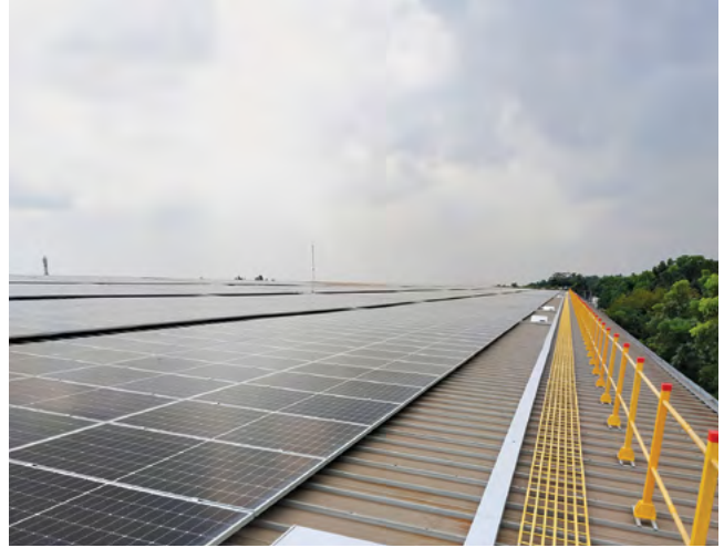
2 MW Industrial Roof Top in Coimbatore, Tamil Nadu
