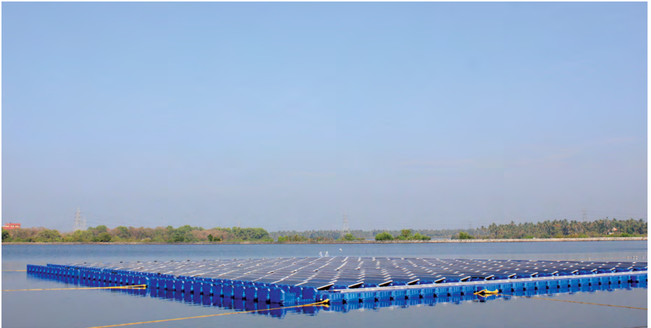
100 kWp Floating Solar Power Plant at Alappuzha District, Kerala
