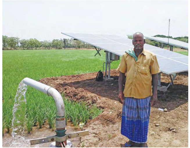
10HP DC Submersible Water Pump at Theni District, Tamil Nadu
