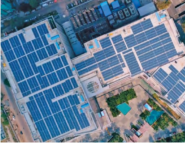
1 MW IT Park Roof Top in Chennai, Tamil Nadu
