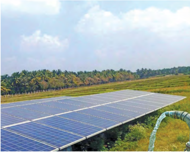
15 HP Solar Water Pumping System, Coimbatore, Tamil Nadu
