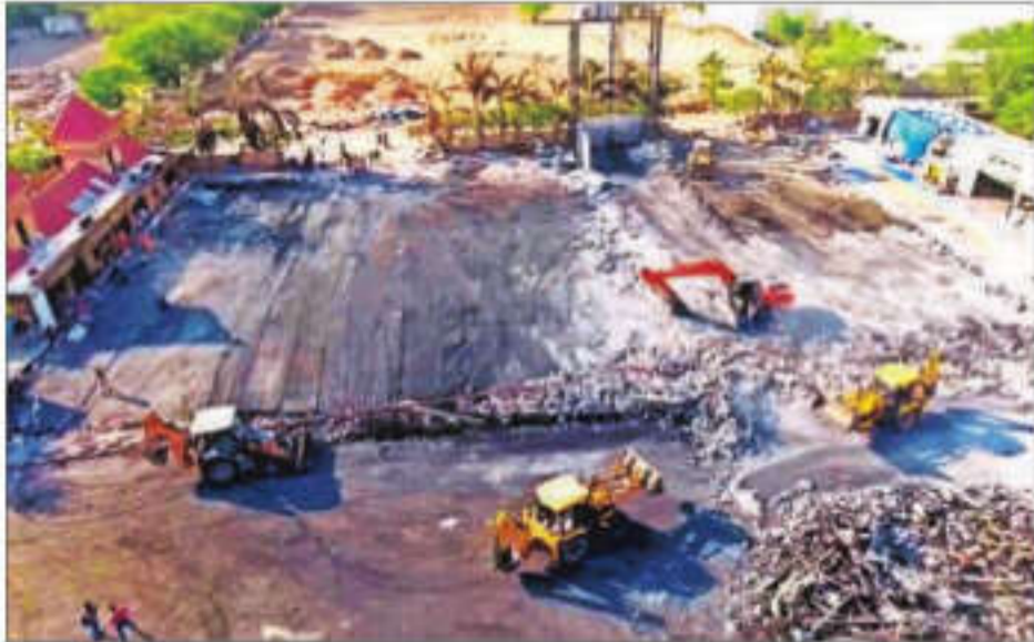
Debris being removed from the game zone site where a fire broke out on Saturday, in Rajkot, on May 27. At least 27 people were killed in the fire, according to officials.
