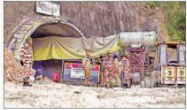
trenchless technique to create a small but stable passage for the workers.
