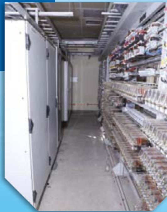
Signalling Equipment Room
