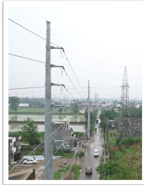
66kV D/C Ckt I & II Lodhawal to GT Road Sub-station
