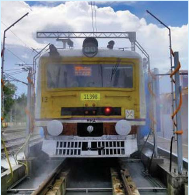
Commissioning of First of its Kind Automatic Drive-through Train Washing Plant at the New EMU Car Shed, Ranaghat, WB on 30th August, 2021.
