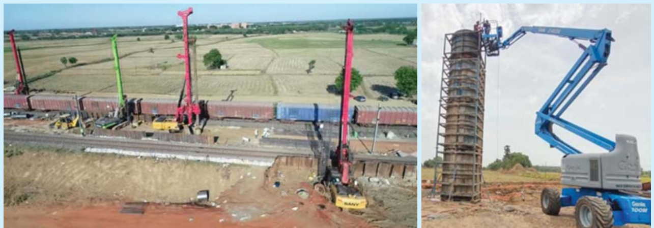
Completion of 525 Piles in Five Months Contiguous to the High-Density Rail Network Near Gudur In Connection with a Rail Flyover Despite Covid Challenges
