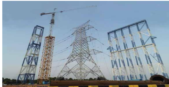
765kV Transmission Tower
