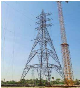
220kV Transmission Tower
