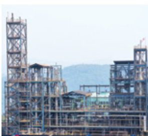
Our IB plant at Lote, Maharashtra
