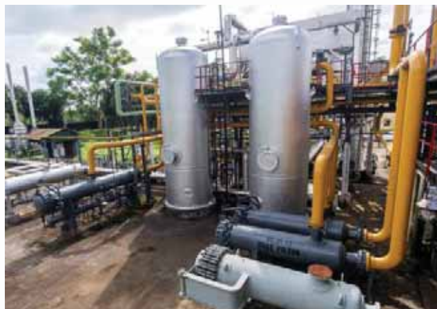
View of a Production Installation at Fields Headquarters
