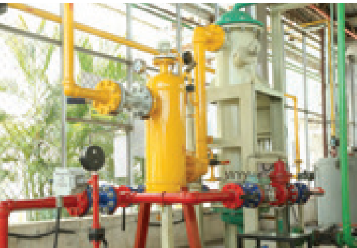
The heater less vapouriser installed at Wada Plant, which has replaced the 36kW electrical heater base vapouriser, has achieved energy saving of ₹5.1 lakhs/annum with a payback of 14 months
