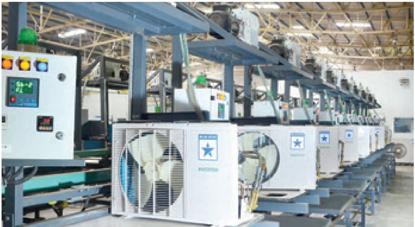
The room air conditioners manufacturing facility at Himachal Pradesh
