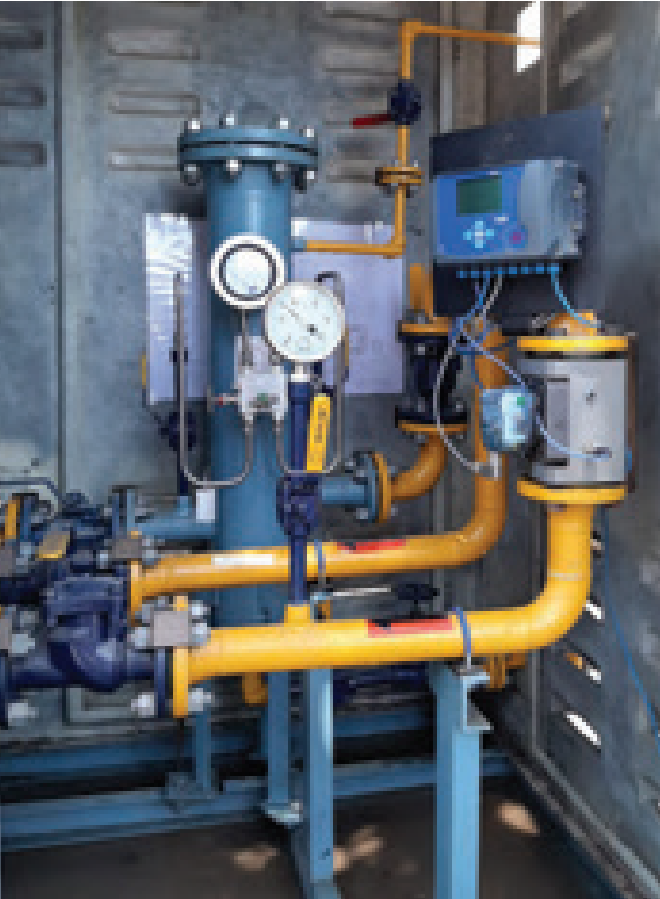
Replaced LPG with PNG for fuel efficiency at Dadra Plant
