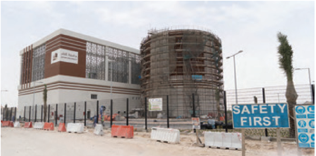
Qatar University project; scope of work - construction of the district cooling plant, including complete civil and MEP works
