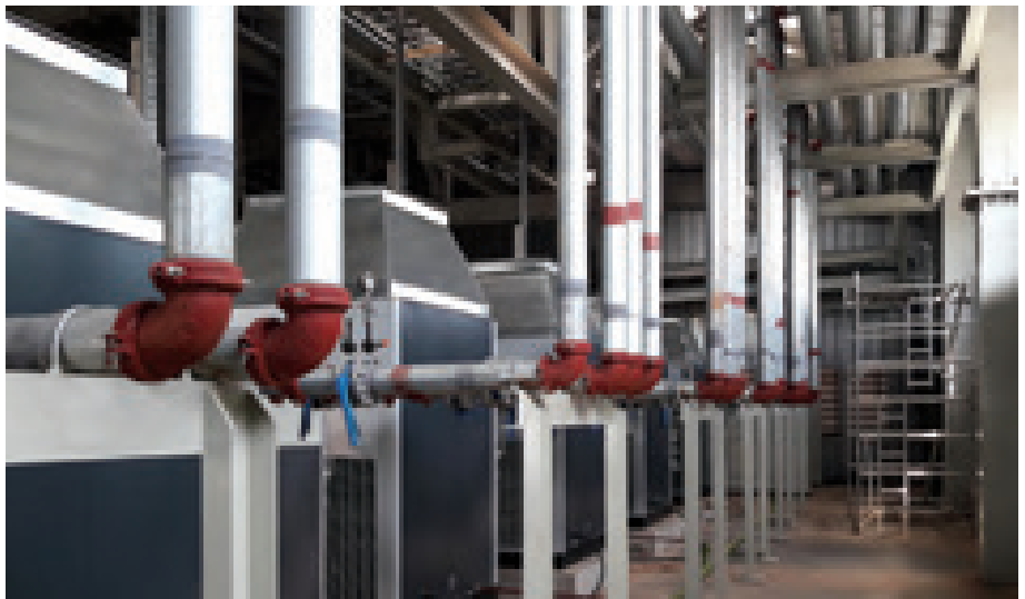
HVAC and Mechanical Piping at Apollo Tyres, Tada, Andhra Pradesh
