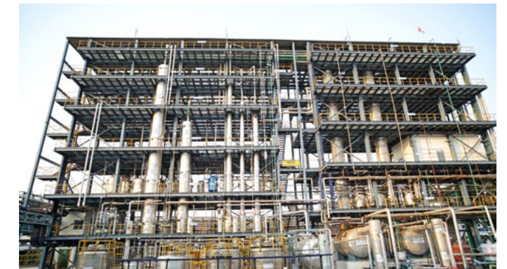
Solvent recovery system
