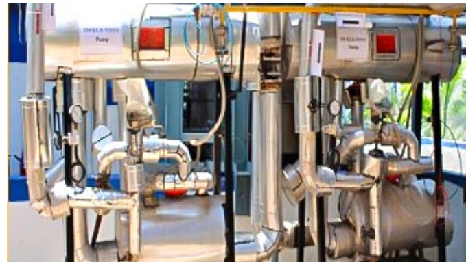
Installed packaged pressure powered pump unit (PPPPU)
