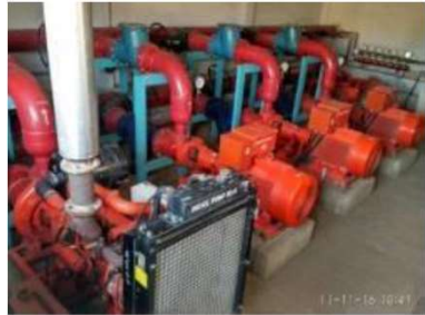
Fire Hydrant Pumps
