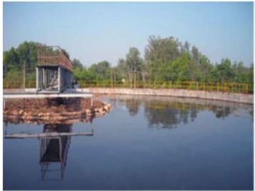
Primary Clarifier - Paper
