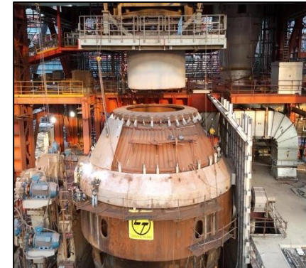
Converter-2 at SMS
