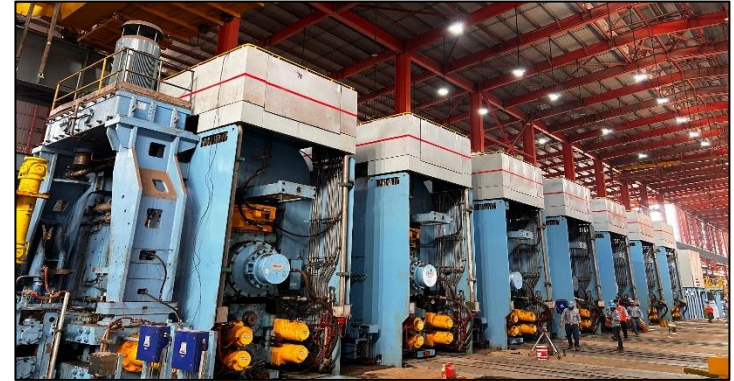
Finishing Mill Stand at HSM
