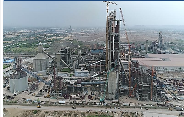
Construction of a 140 m tall Preheater & 40 m wide Clinker Silo for a Cement plant
