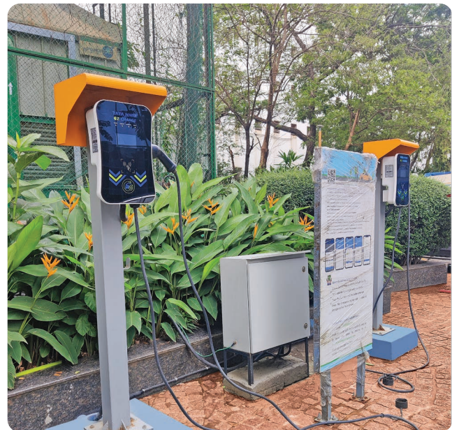
The charging station for electric vehicles at ICICI Service Centre in Bandra-Kurla Complex, Mumbai.
