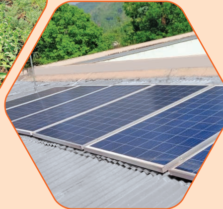
Solar panel installation in a school at Mawbri village in Ribhoi district, Meghalya.
