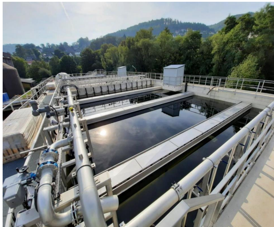
Altena WWTP, Germany
