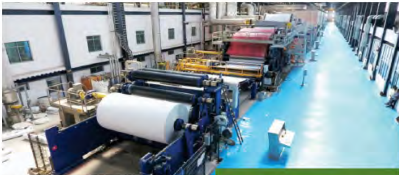
Board Machine in TNPL Board Plant - Unit II
