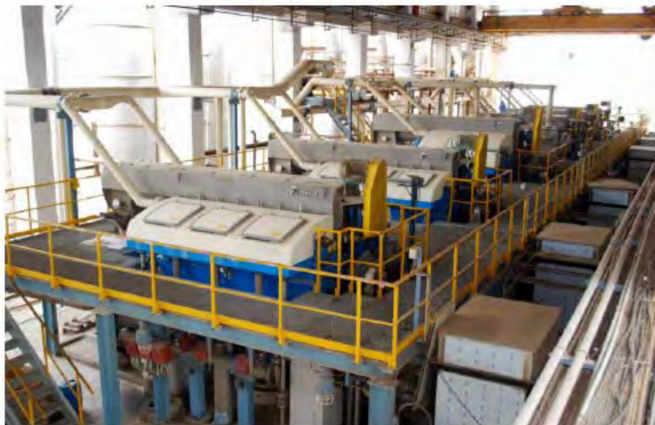
Elemental Chlorine Free (ECF) Bleaching Plant
