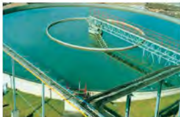
Waste water treatment plant
