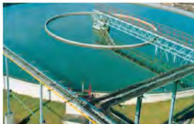
Waste water treatment plant
