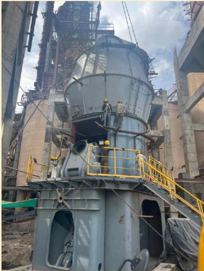
VRM (Cement Grinding) Completed...
