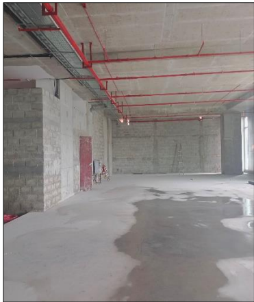
Internal View of the SP
