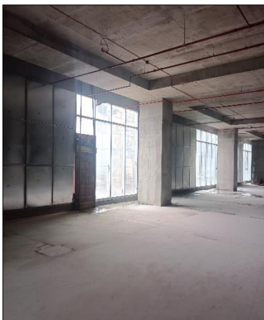
Internal View of the SP
