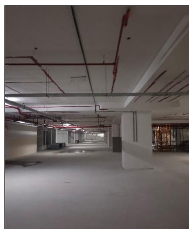
Internal View of the SP
