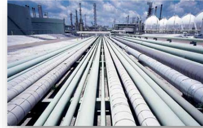
Anti Corrosive Material
