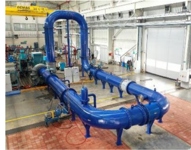
FGD pumps testing set-up
