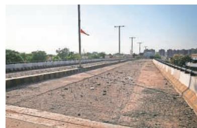
Hatkeshwar flyover was closed for public use due to the damage caused to it. File
